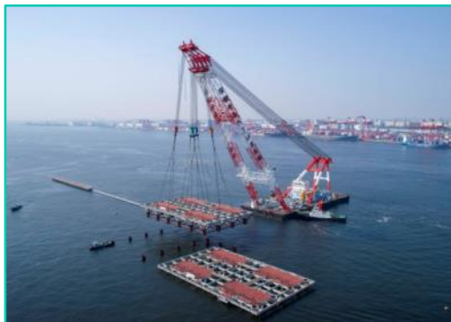
Construction zone #13 for new passenger boat wharf, quay, and parking area, etc.
